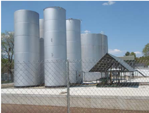
Figure 1. Bulk Petroleum Storage
