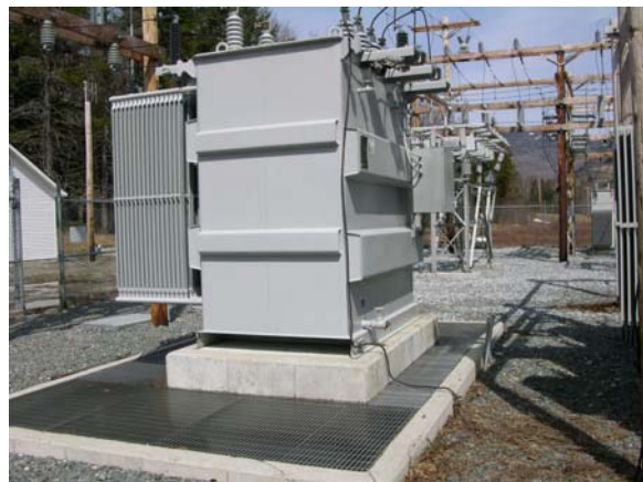
Figure 3. Transformer with Secondary Containment
